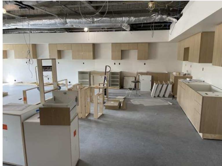
Raytown HS FACs Room Installation
